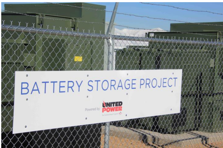
United Power began use of a Tesla battery packs in December 2018 along I-25 north of Denver, but did so in a conflict with Tri-State Generation and Transmission.
