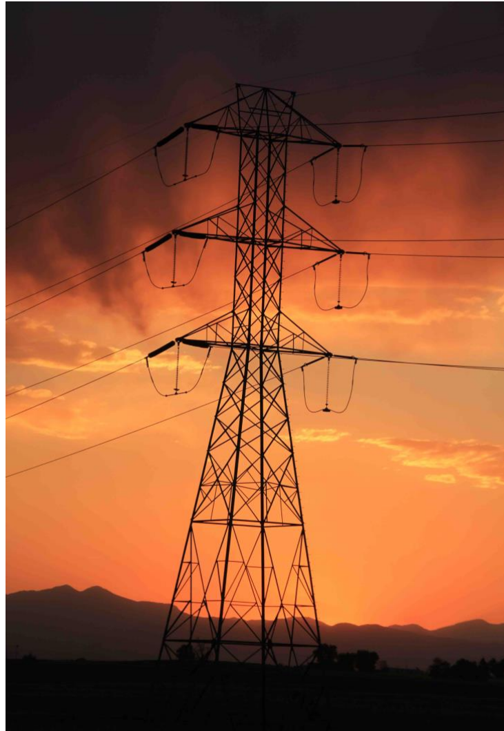
A transmission tower near Firestone, north of Denver, an area served by United Power and its wholesale supplier, Tri-State Generation and Transmission. Photo/Allen Best
