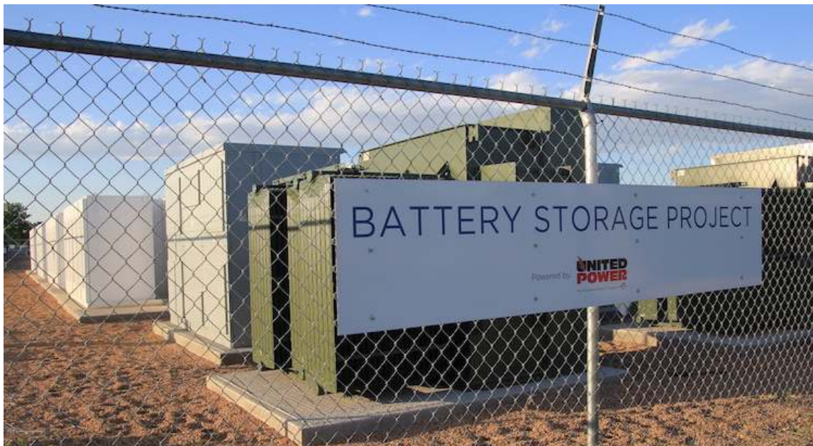
The battery storage United Power put into service in late 2018 has been a point of friction between the cooperative and its wholesale supplier, Tri-State Generation and Transmission. Photo/Allen Best
