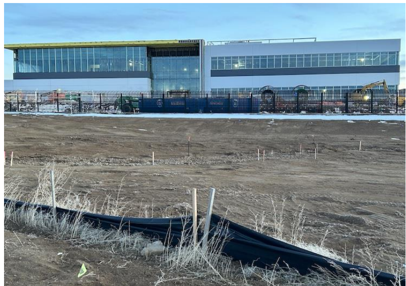
Construction of the QTS Data Center in Aurora appears to be well along the way to completion. Photo/Allen Best
