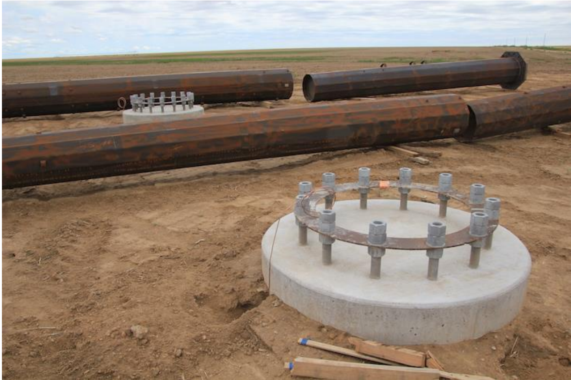
Two of the five segments of the Colorado Power Pathway 345-kv transmission line are well along the way toward completion. Above, foundation south of Cheyenne Wells ready for a tower to be added. And at right, the line near Sheridan Lake seemingly completed but not yet energized.
